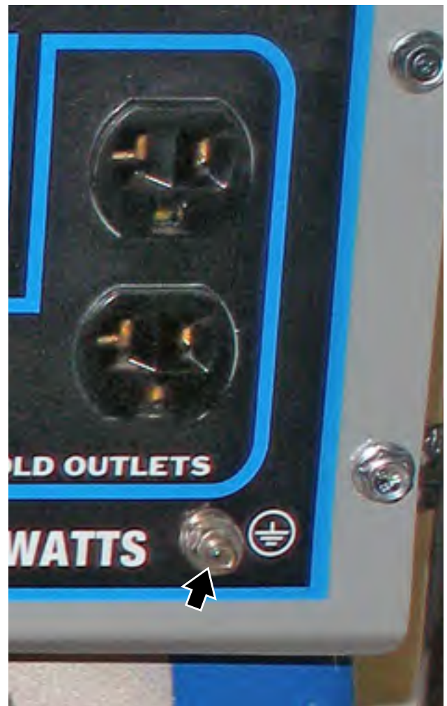
Figure 12 – Ground Terminal on the Control Panel
